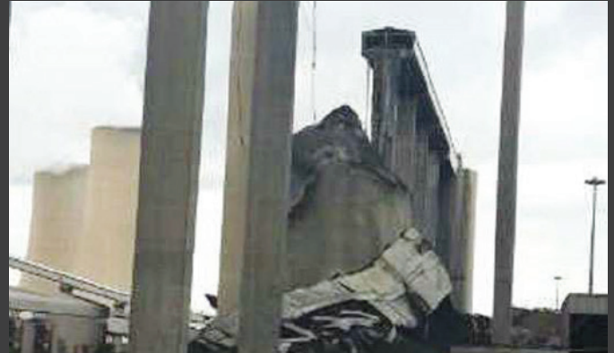
Collapsed silo at the Majuba Power Station. Source: Andriesvanheerden.wordpress.com
