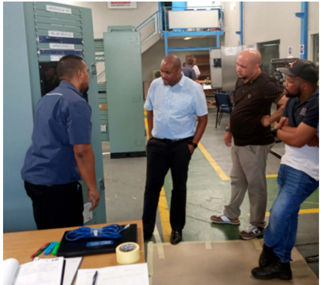
Factory Acceptance Testing of Human Machine Interface panels, March 2023. In the centre, Mr Duma Mhaule Director: Electrical Engineering Services, and the KDM Project Manager Mr Brendan Pillay on left, with staff from Control SI, illustrating the built components and their operations.
