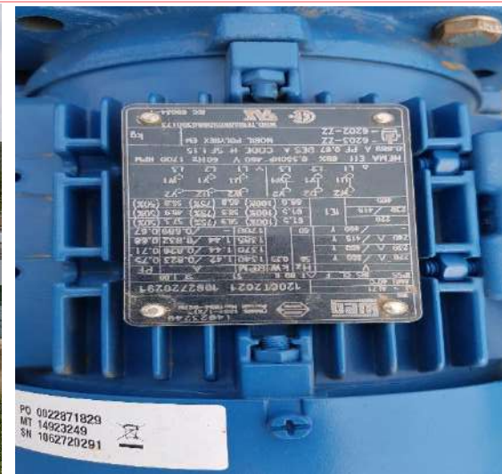
Motor operated water clarifier.
