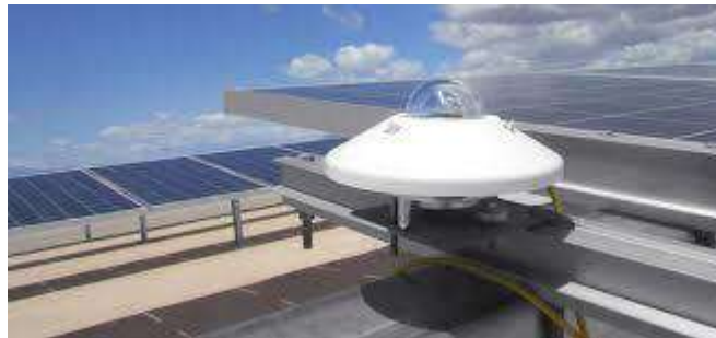
Figure 34: Typical inclined Kipp & Zonen Pyranometer
