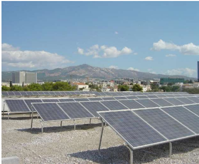
Figure 4: Rooftop PV installation example
