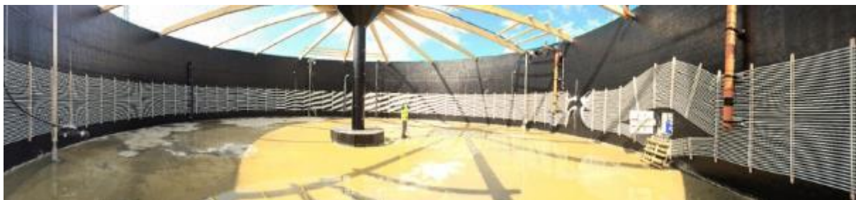
Figure 19 Digester with water heating pipes from Thermophilic process
