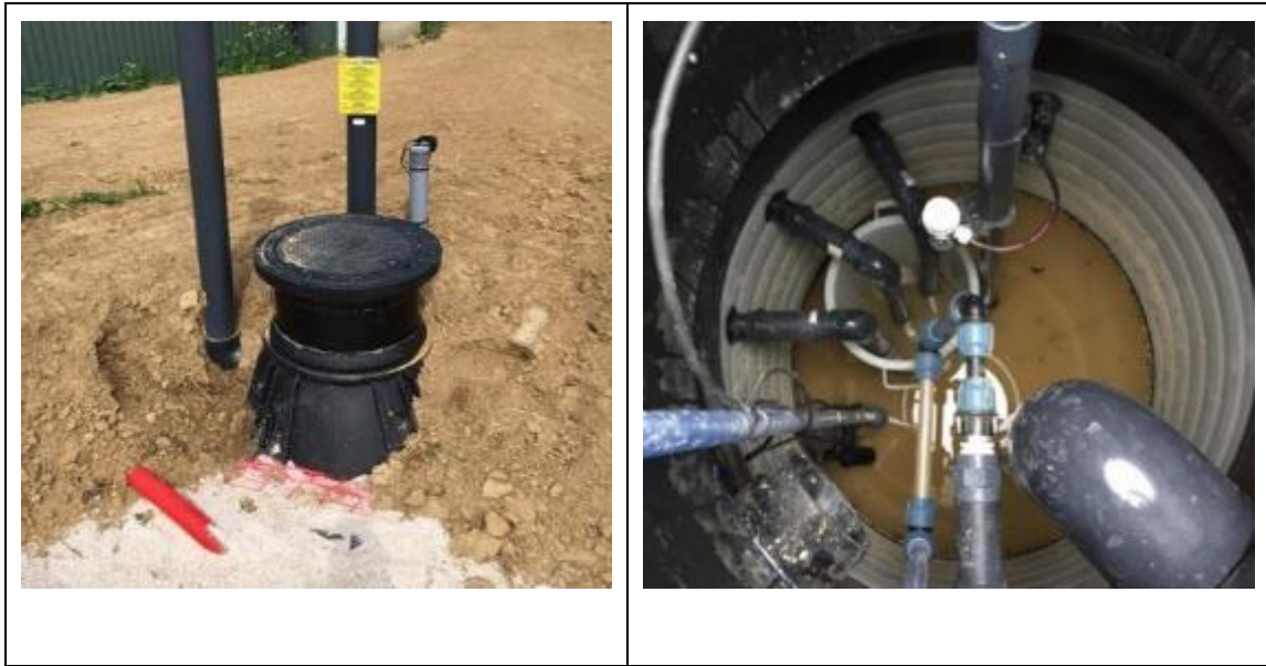
Figure 26: Digester Condensate removal system
