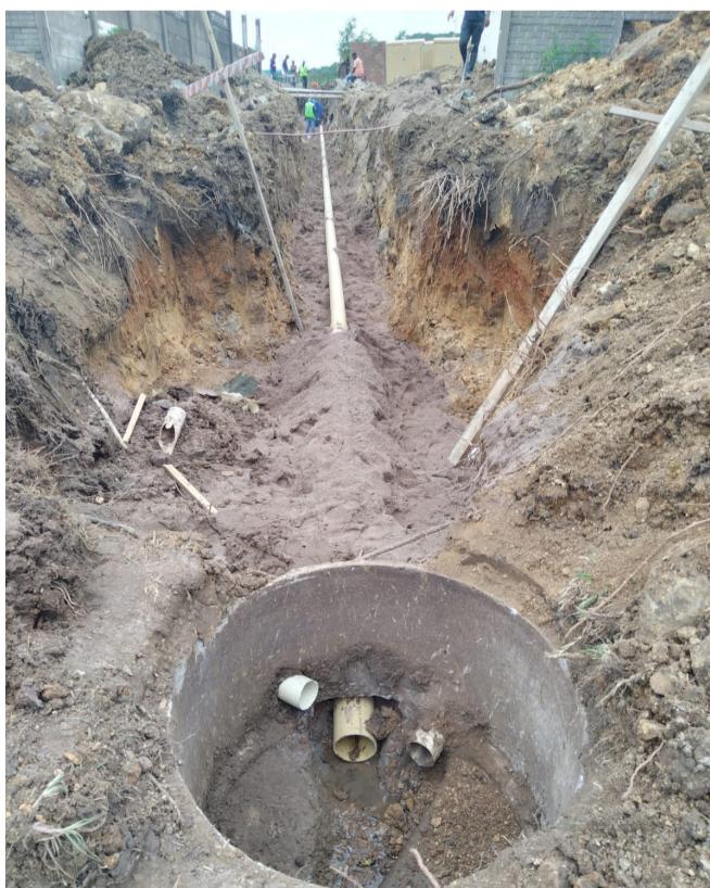
ThakasaQ Trading Enterprise installed new sewer line for the new offices of Mandeni Drivers License Testing Centre
