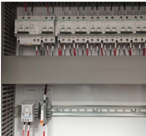
Elements of the neatly-designed and manufactured panel components to record and communicate real-time information on the substation's operations at and between the local SCADA and master SCADA at the Control Room.
